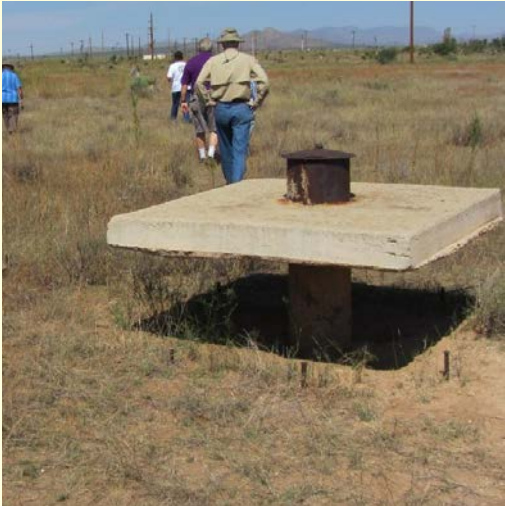
Subsidence, leaving well head exposed above ground (Above)
