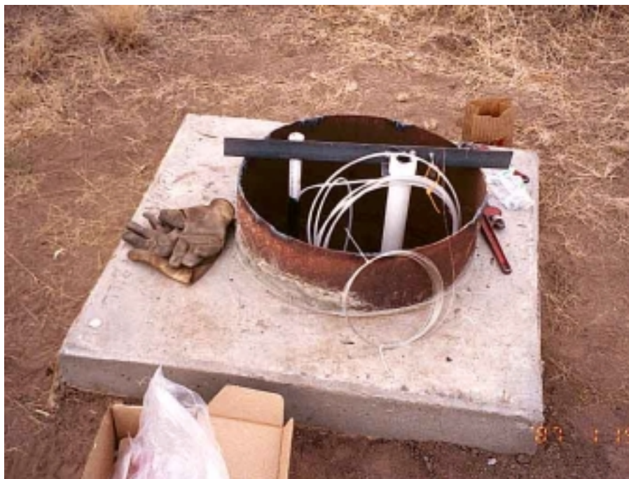
Figure 5. Surface hanger supports data logger
